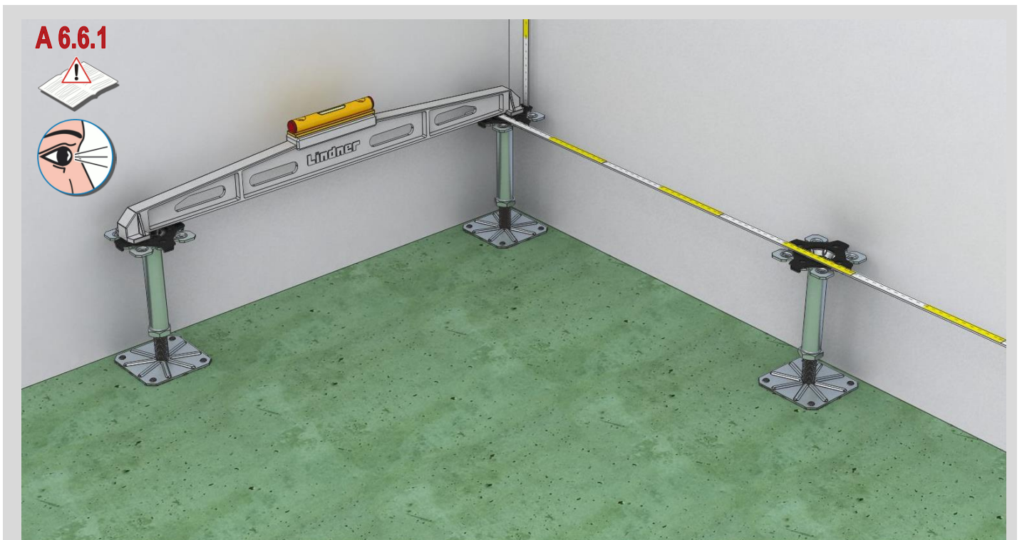
Picture 13 Installation of the following pedestals for the first raised floor panel
