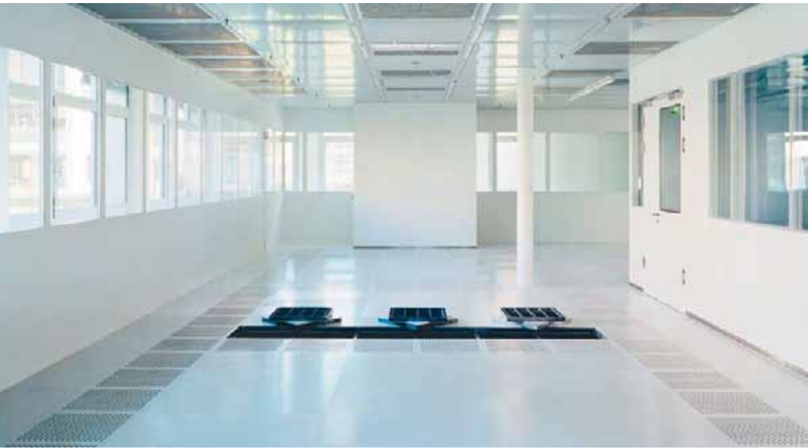
Infineon, Munich – Lindner installed the ceilings, floors and walls as well as the lock control system.
